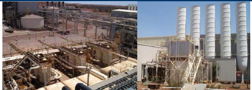
Figure 1: SX-EW plant purchased from Cawse
